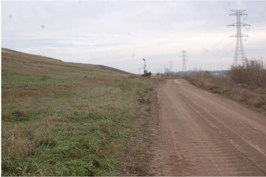
Photo 51 - Cell 2B/2C South Perim Rd/LF Toe
