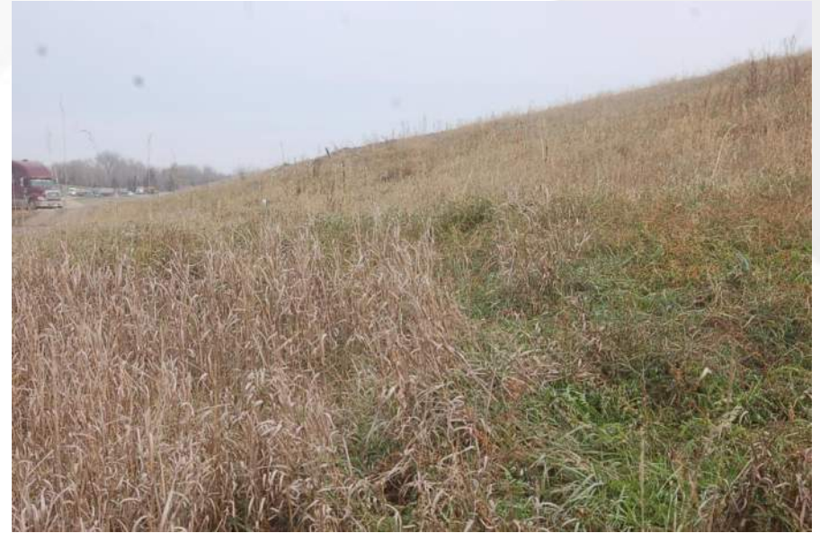
Photo 64 - Cell 2A West Landfill Face
